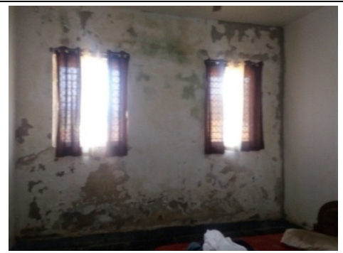
Picture 2.7: Seepage in wall of WSA Trikut, Deoghar
